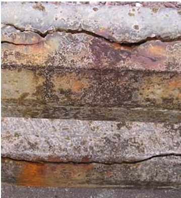
Typical longitudinal concrete cracking and staining due to reinforcement corrosion.
