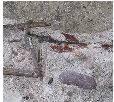
Severe localized corrosion and complete loss of reinforcement, without visible external damage.
